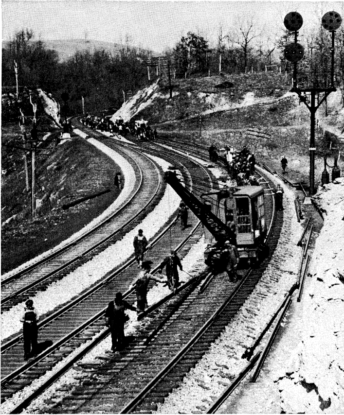
Rail-laying gang in action on a U.S. railway. Rails are lifted into place on wooden ties by derrick. Other units following align the rails, join rail sections and drive spikes into tie plates
