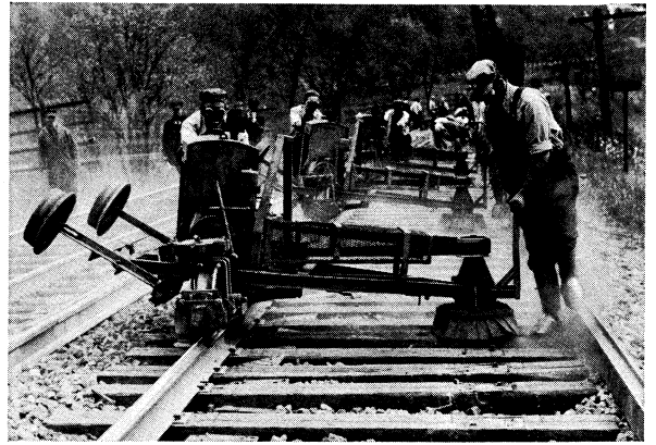
Adzing machines, which cut a uniform seat for tie plates before new rail is laid
